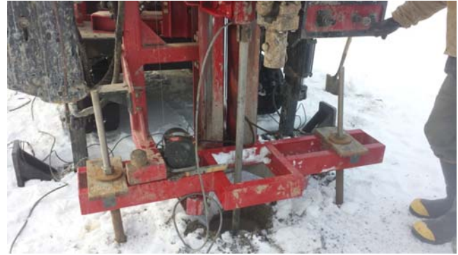
Figure 6-2 Photograph of AMS dual anchor with pre-drilled pilot hole augured through frost
