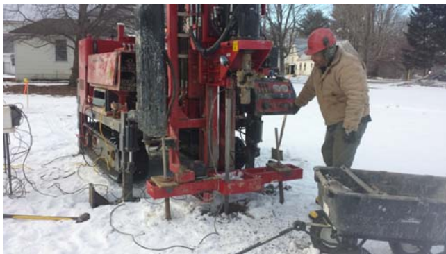
Figure 6-1 Photograph of SCPTu performed with AMS PowerProbe ® and Vertek VTK cone system
